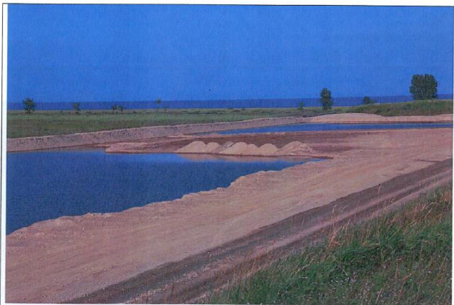
Description: North Berm and Backfill Area at East Central End of Industrial Canal (Facing Northeast) Location: Johns Manville Site, Waukegan, IL Date: July 30, 2014
