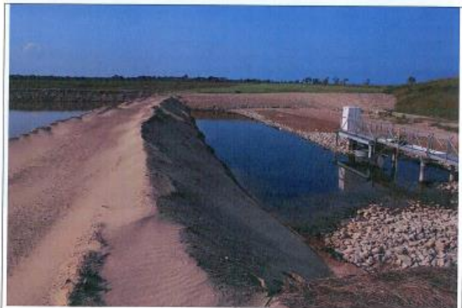
Description: Sand Isolation Berm at East End of Industrial Canal (Facing North) Location: Johns Manville Site, Waukegan, IL Date: July 30, 2014
