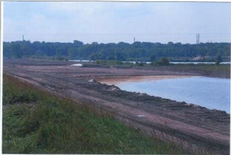
Description: Backfill Area at West End of Industrial Canal (Facing Northwest) Location: Johns Manville Site, Waukegan, IL Date: July 30, 2014
